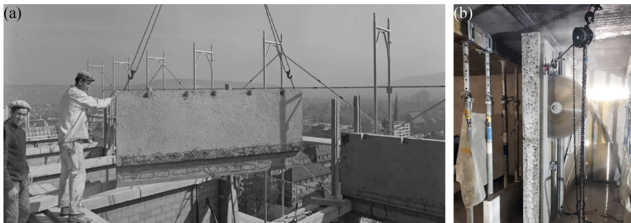
Fig. 1. (a) Careful construction of prefabricated RC structure in 1964 and (b) sawing of an existing RC wall. Image credits: (a) Baugeschichtliches Archiv (BAZ) Stadt Zürich, Köhli Ernst; (b) Diamcoupe S.A.
