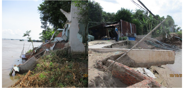
Fig. 2: River bank erosion in the upper part of the VMD
