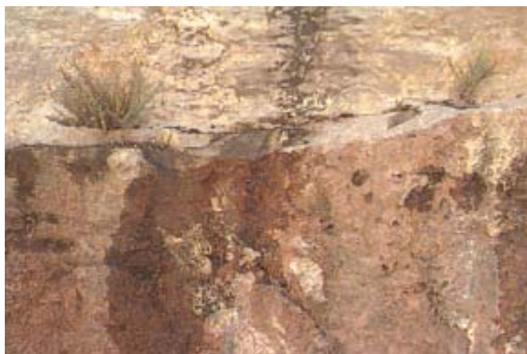
Figure C.6 Photo of wet spots. Water seeps from a bedding plane and from some spots where the fractures are not directly visible.
