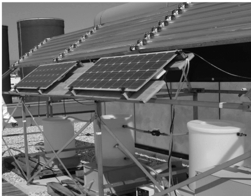
FIGURE 5.4 Coupled solar-biological flow reactor at pilot scale installed at EPFL.
