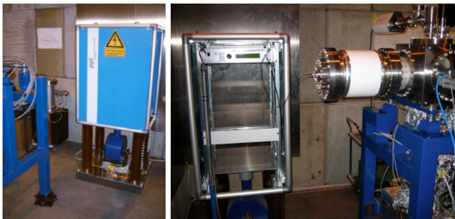
Figure 4.8: The hotdeck consisting of a 19" rack that holds the gate pulser and electronics for communication (in the rack) as well as the 230 V isolating transformer (between the rack and the base). The cathode flange with the SMA vacuum feedthrough, ceramic insulation and diagnostics cube are shown in the right picture.
