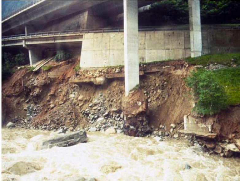
Figure 1.2. Undermining of a bridge pillar (from Loat and Petrascheck, 1997)
