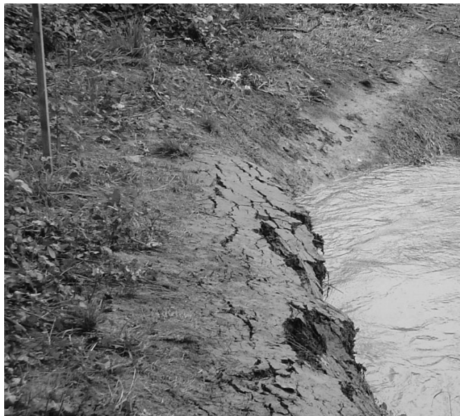
Figure 4.14. Observed tension cracks at bend 3.3 during the drawdown of the October 26, 2004 flood
