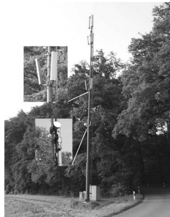
Fig. 3.4b: Example of GSM BTS well-integrated into the landscape by colouring the mast in green (near Winterthur (CH)).
