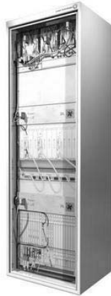
Fig. 3.8: NodeB rack (Lucent Macrocell Indoor; picture provided by courtesy of Lucent Technologies).
