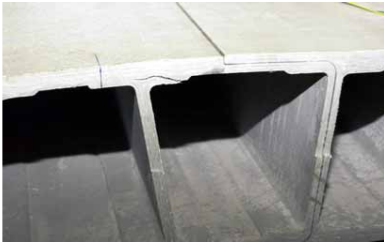
Figure E.26: Crack due to secondary bending moments in the upper face sheet, axis G - G
