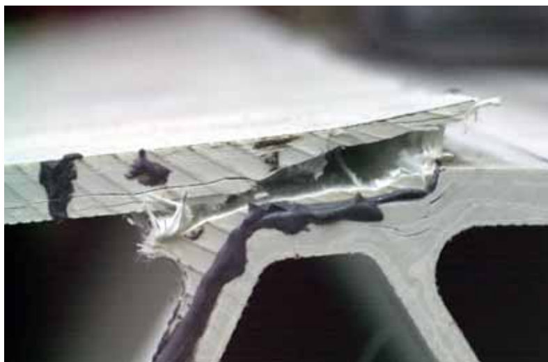
Figure E.16: Detail failure of upper face panel, axis H - H, back view
