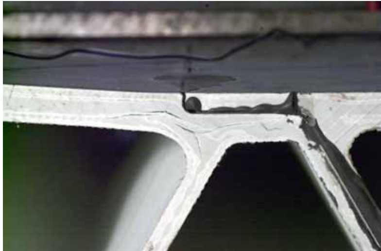
Figure E.21: Small cracks near location of failure, axis L - L
