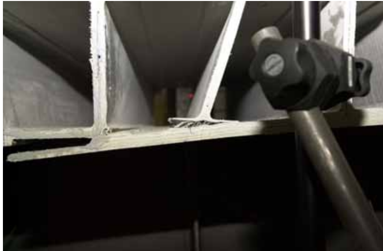
Figure E.23: Front view with failure in axis H - H
