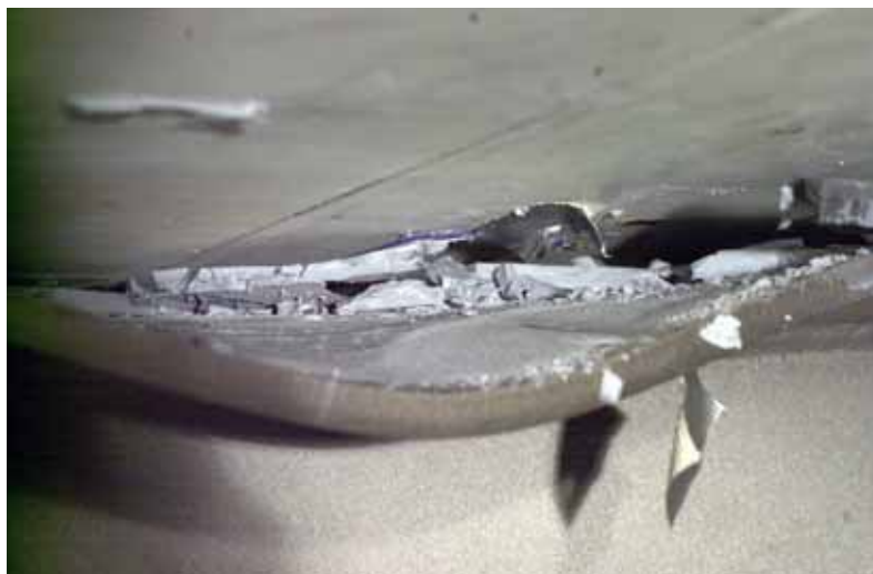
Figure 4.36: Detail adhesive bond after failure, back view axis J - J (The failed adhesive was taken away for the photo)
