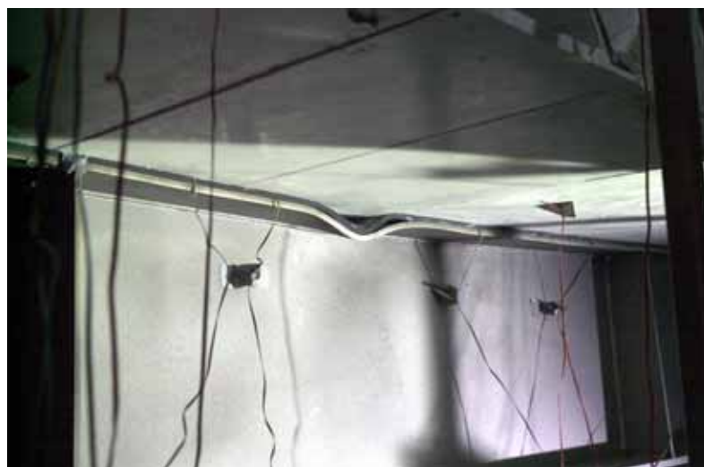
Figure 4.35: Local detachment of deck at mid-span and buckling of top steel flange, girder Fix 4.
