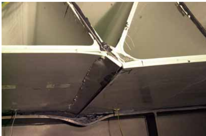
Figure E.11: Under view of axis K - K with buckling of top steel flange at location with detached bridge deck
