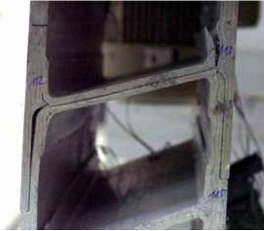
Figure 3.39: Web delamination and joint failure (specimen 3ca)
