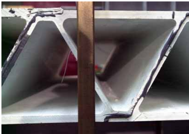
Figure 4.30: First and second failures in the upper and lower deck panels near axis H-H, girder Fix 4.
