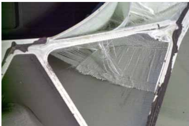
Figure E.8: Failure axis G - G with delamination of inner mat of the upper face panel
