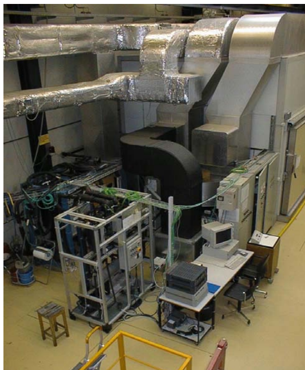
Figure 2.17: Two-stage compression heat pump tests with an air-water test section, climatic air is produced in a separate circuit including the Igloo (big room at the right hand side of the picture).
