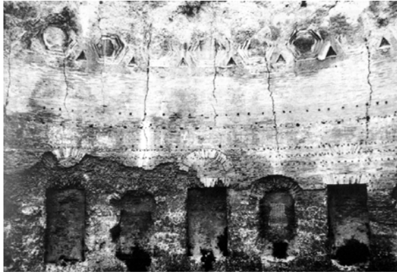
Fig. 28: (a) Cracking around the base of a concrete semi-dome, Baths of Trajan, Rome. (Mainstone 1 )
