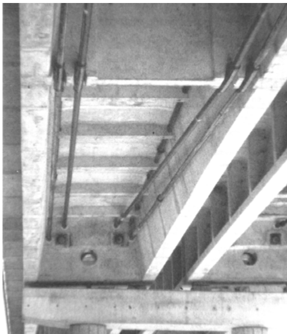
Fig. 70: Pi section, open from below with external prestressing. Saint-Agnant Viaduct. (SETRA, after Freyssinet)
