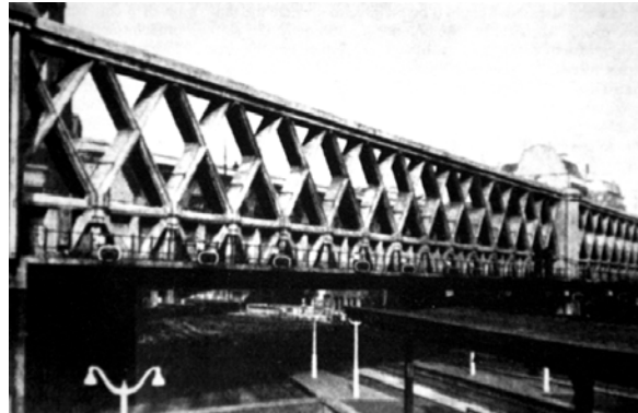
Fig. 10: Trussed reinforced-concrete bridge, the Rue Lafayette Bridge over the railway lines at the Paris-East Railway Station with a span of 71.87 m and a depth of 10.40 m, Caquot, 1928. (Deinhard)
