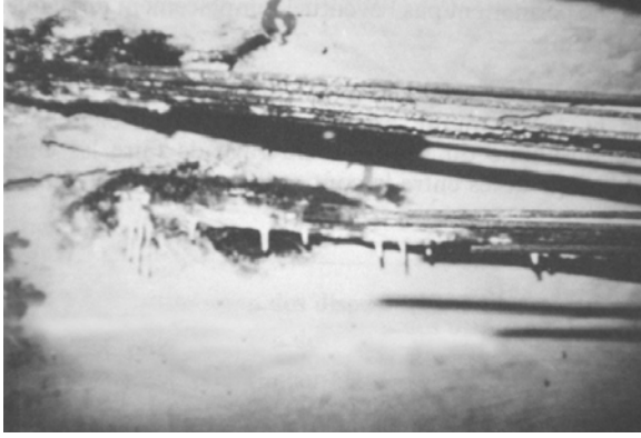
Fig. 66: Corroded and ruptured cables of the Can Bia Bridge. (AFPC et al., after J. Châtelain)
