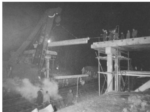
Fig. 40: Erection of precast prestressed concrete girders over railway tracks in Germany to construct a field access bridge. (Wittfoht)
