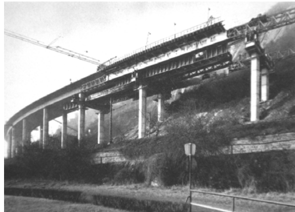
Fig. 49: Krahenberg Bridge, first prestressed concrete bridge built using span-by-span cantilever construction method with self-supporting traveling formwork. (Wittfoht)
