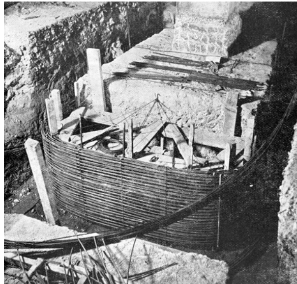
Fig. 19: Prestressing system used by Freyssinet to jack the tendons of the tie beams in the Gare Transatlantique at Le Havre, 1934. (Freyssinet)
