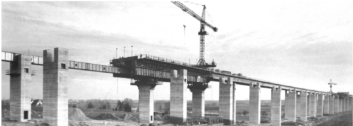
Fig. 46: Example of traveling girders that support formwork from below the bridge deck. Note the openings provided for at the top of the piers to allow the traveling girder to pass. Image shows the construction of the 1.5 km Pfeddersheim Viaduct for the A 61 between Ludwigshafen and Krefeld, Germany. (Wittfoht)
