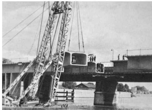
Fig. 57: Segment of the Choisy-le-Roi bridge being placed with a floating crane. (Podolny and Muller)
