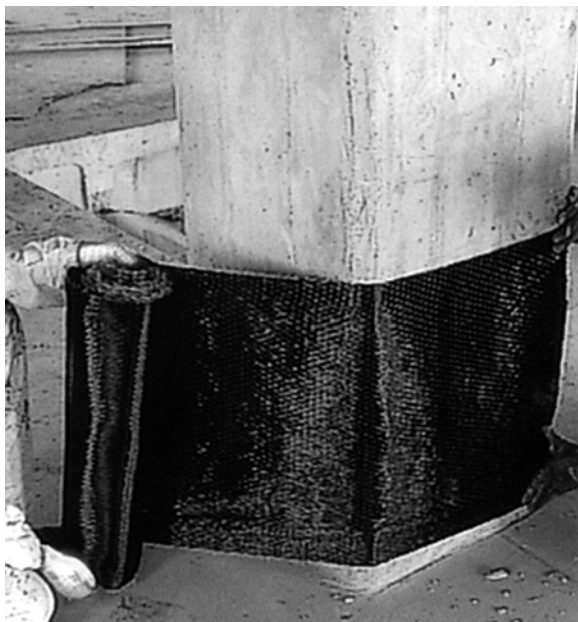
Fig. 6.18: Example of FRP sheet reinforcement of existing reinforced concrete bridge pier. (CCLab, after Sika)
