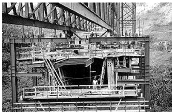
Fig. 4.39: H-3 North Halawa Valley viaduct, Oahu, Hawaii. Cast-in-place form traveler construction. Parsons Brinckerhoff Hirota Associates, 1996. (Sanders)
