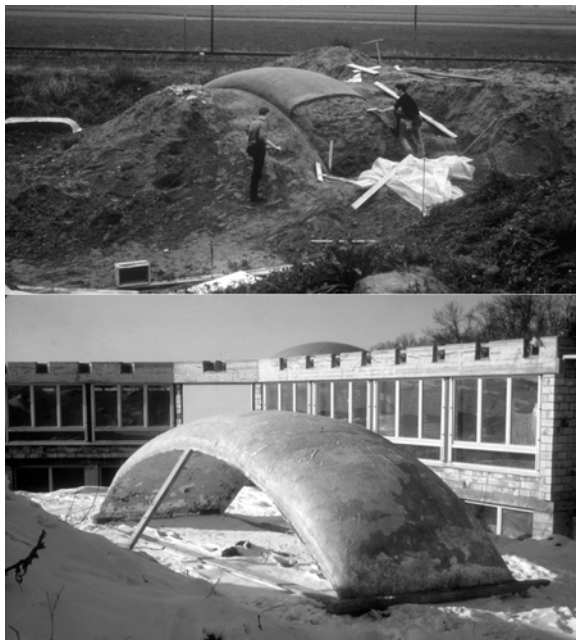
Fig. 4.24: Example of the hand lay-up method of producing complex FRP component. In this case the mold was formed with earth, however better quality can be attained in factory conditions.
