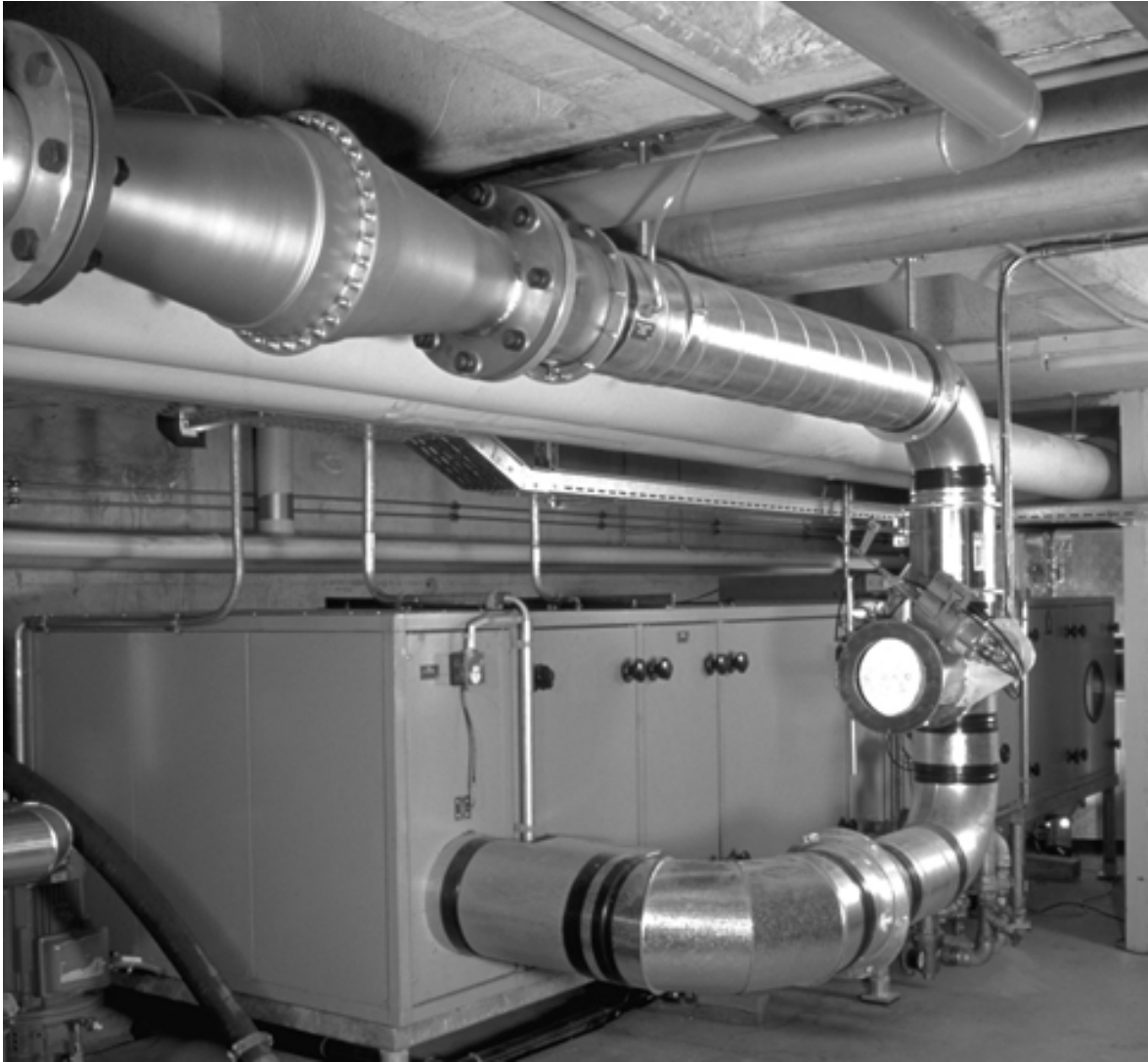
Figure C.4: Air conditioning system and laminar flow meter installed on the piping.
