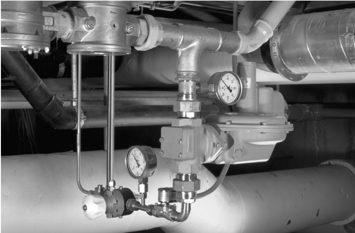
Figure C.5: Compressed natural gas expansion system: 40 to 5 bar (bottom, left), 5 to 50 mbar (middle, right) and connection to the network supply.
