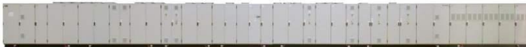
▲ ABB's ACS6000 multi-drive line up - around 33 meters long - modular design done 20 years ago!
