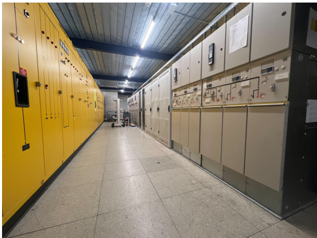
▲ PEL Low Voltage and Medium Voltage switchgear
