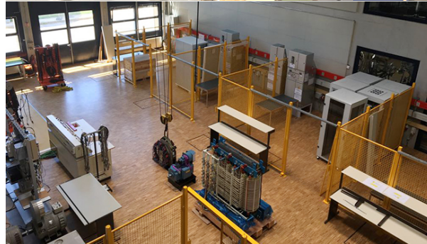
▲ MV Power Electronics Laboratory
