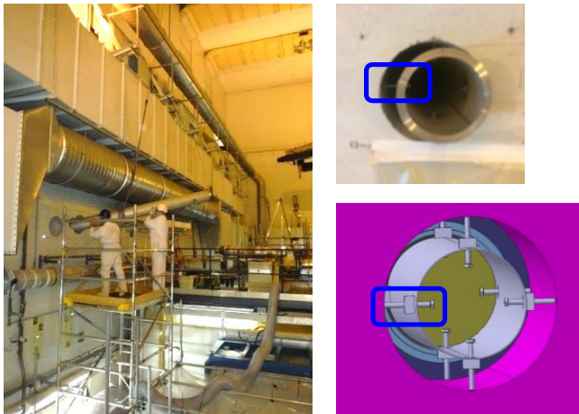
Figure 67 Left: Photo taken during the installation of the WAV penetration tube. Right: Photo and model of the alignment adjusters used during the alignment of the penetration tube.
