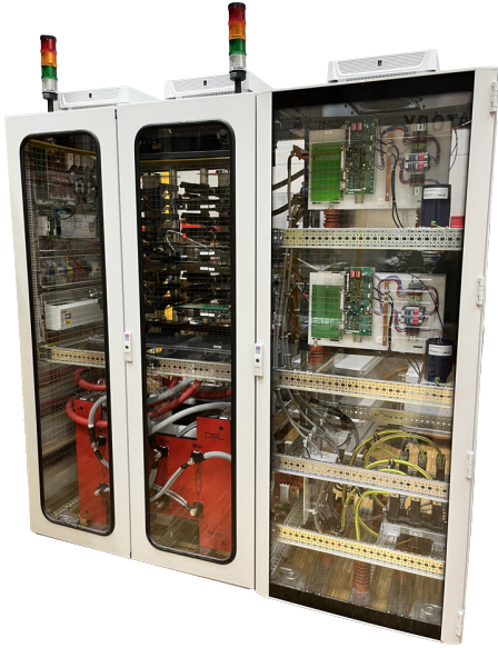
Fig. 2. Photo of the 1 MW MV DCT prototype.
