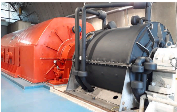
Fig. 3. generator (red) and flywheel (black).
