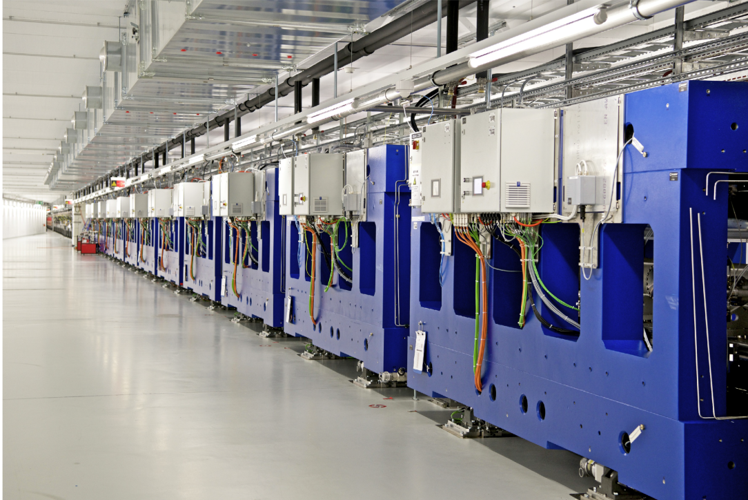
Figure 3.4: Aramis undulator at SwissFEL. The Aramis undulator is 60 m long, with a 4 m length for each module and 0.75 m for each intersection [3].
