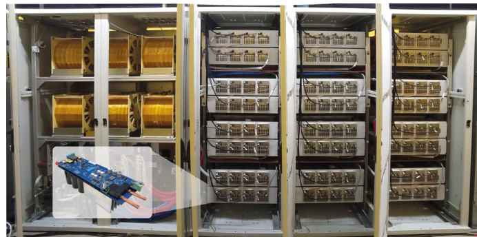
▲ EPFL PEL - Dual MMC-based MVDC source - realized 2 x 250kW system
