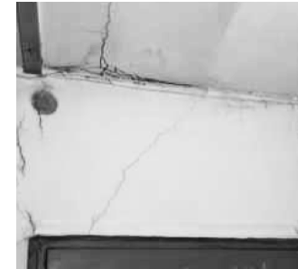
Visible cracking on joints
