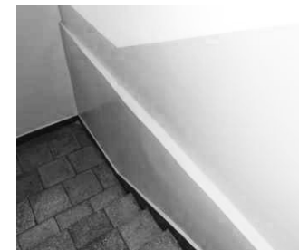
Assembly errors, no common wall axis.
