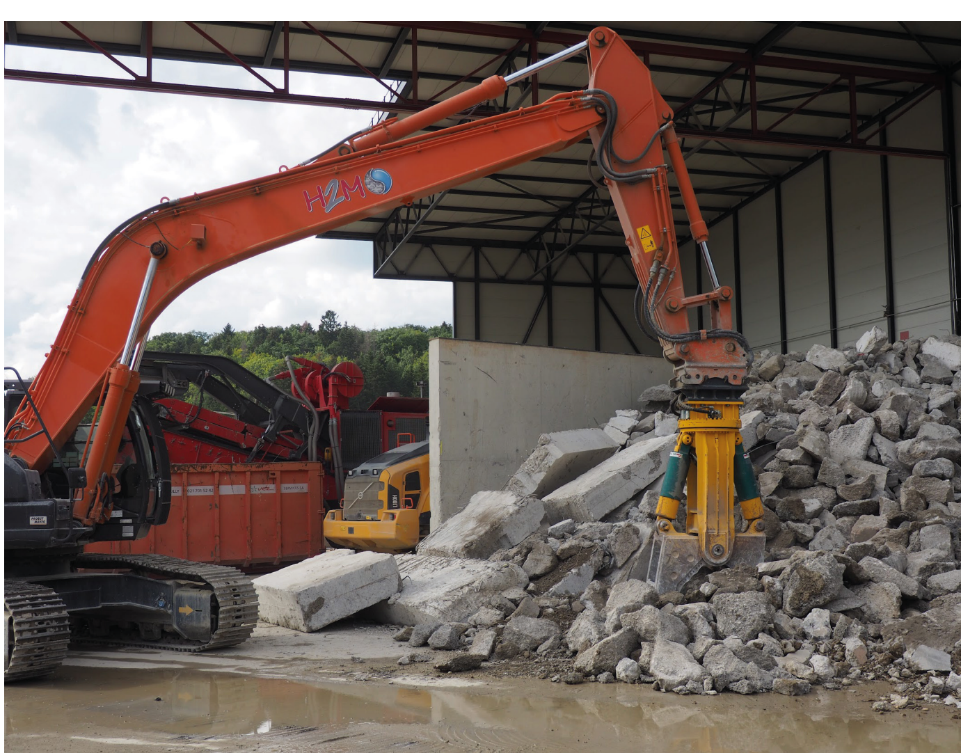
Tools and processes involved in the end of life of reinforced concrete
