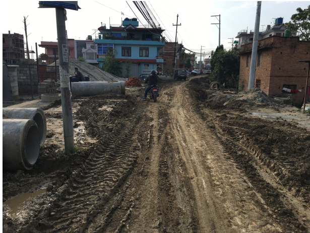
Figure 30: Type A: Road under construction in Duwakot with stormwater drains considered as a sewer system
