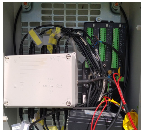
Figure 2.5: Data network box
