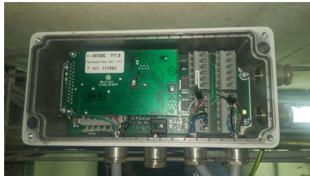
(a) Junction box, VKK1-4, HBM
