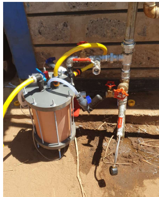
Figure 16: BlueTap chlorinator, Mumo wa Ikaaie.
