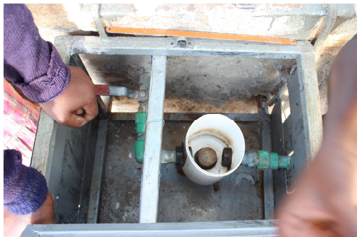
Figure 14: AkvoTur chlorinator with cage, Kitumbini.
