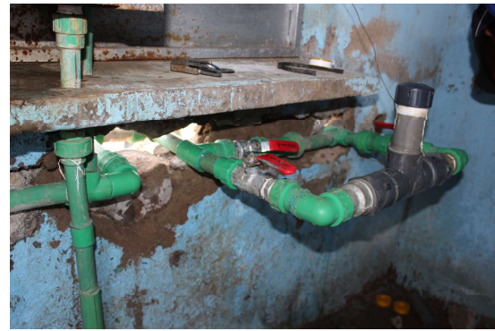
Figure 31: Chlorination system inside the kiosk, Kivui.
