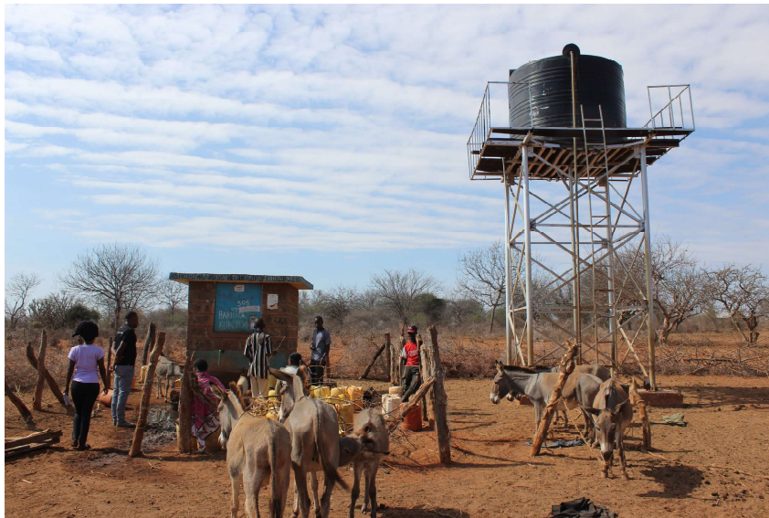
Figure 17: Water kiosk and tank, Ivonyanga.
