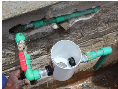
Figure 36: AkvoTur chlorinator installed after the valve.
