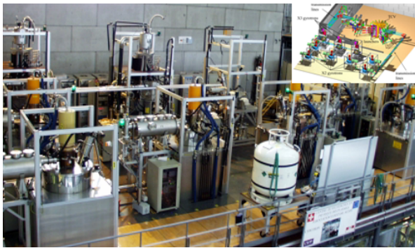
Fig. 9: Image of the TCV's 4.5 MW EC HCD system [86,87], which is located ~30m from the tokamak center (inside concrete wall). A reference of the plant layout is illustrated in the upper right insert.
