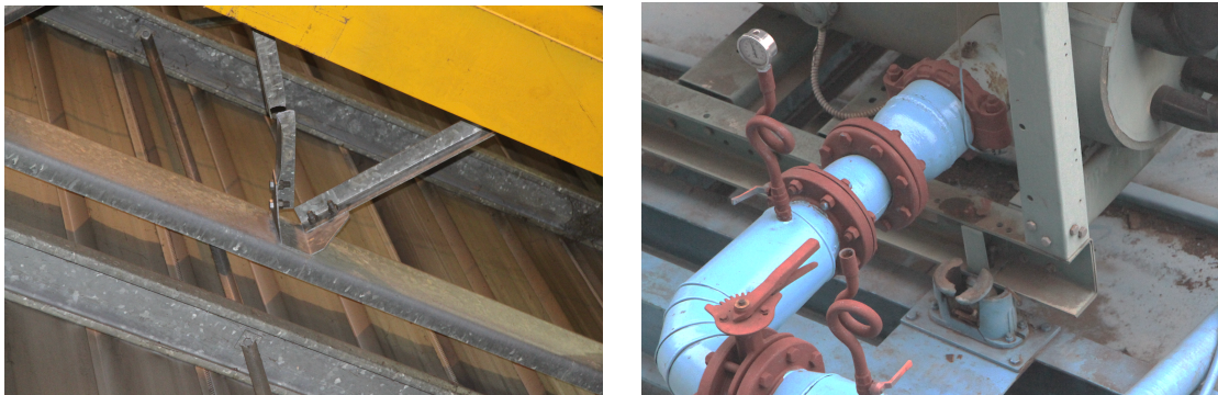
Figure 1. Examples of nonstructural elements that had bracing elements with seismic design but nevertheless experienced failure during an earthquake (Photos by Eduardo Miranda).
