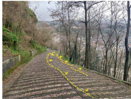
Figure 6. Scarps along the road on the northwest part of the castle. The retaining wall, as well as the lamppost, are rotated and have sunk with respect to the road. In yellow, dotted lines marking shape and direction of deformation on perimetral road below the castle.
