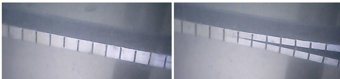
Figure 3: Image recordings with initial crack visible on the left and after crack progression on the right
