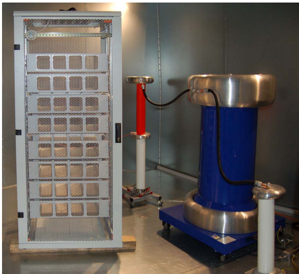
▲ Cabinet of one phase-leg (32 cells) in Faraday cage during insulation coordination testing
