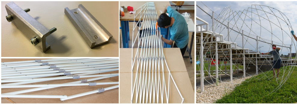
Figure 6: Assembly and deployment of the X-Shell pavilion. The aluminum connecting sleeves (upper left) are used to join the separately-assembled scissor linkages of GFRP beams into the full assembly (bottom left, middle). A preliminary manual deployment (right).
