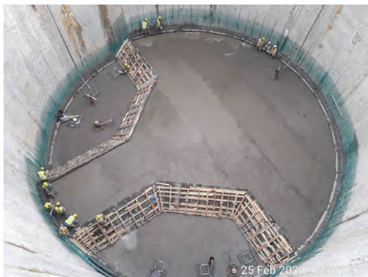
Figure 10: Al-Salam Storm pumping station wet well in construction in February 2020 (photo courtesy Abuljadayel Co. for Cont. & Maint.)
