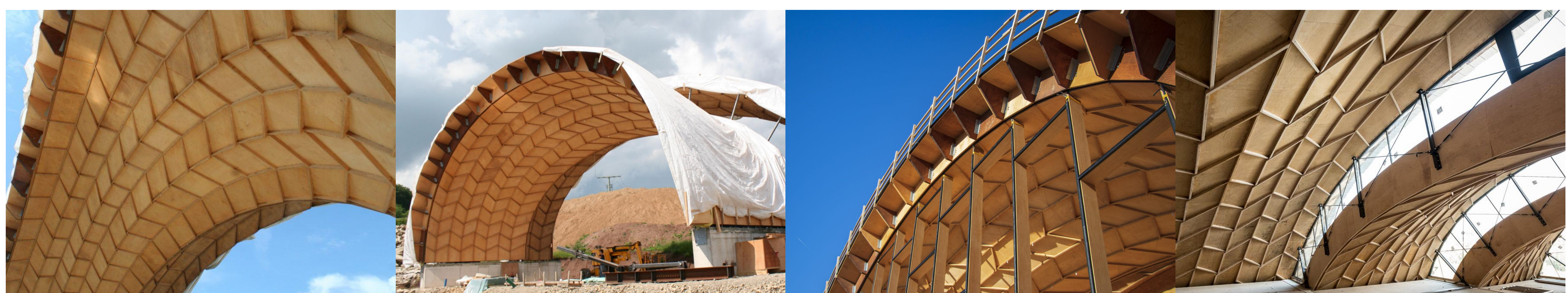
The multipurpose hall of Annen, currently under construction in Manternach, Luxembourg (Architects: Valentiny hvp architects and Yves Weinand, Technology transfer: IBOIS)
