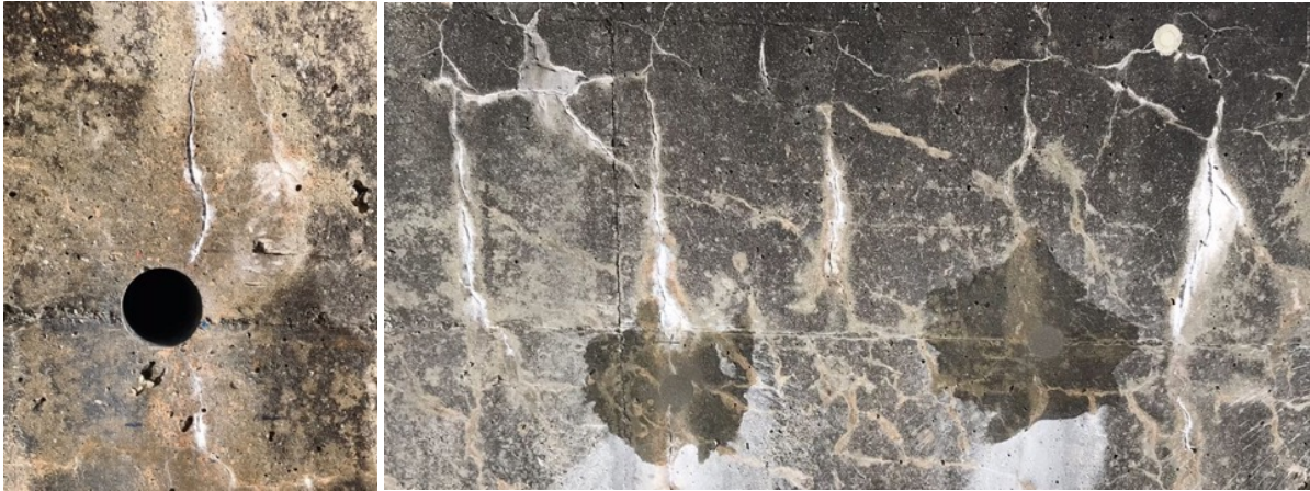
Figure 1.2 : ASR clefts (macroscopic level) in a retaining wall from Brünig area, Bern, CH.
