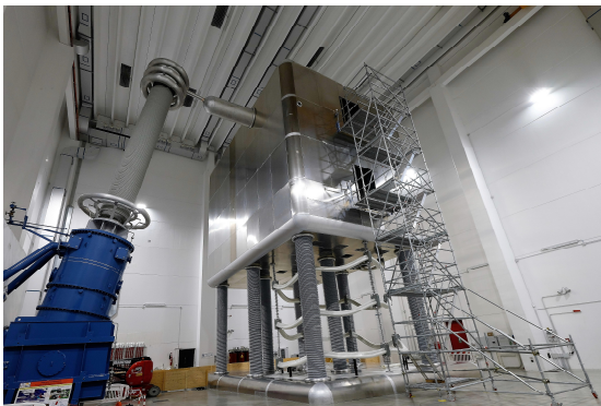
Fig. 7: View of the HVD1 hosting the ion source power supplies and the HV bushing of the 1MV insulating transformer feeding the ISEPS.
