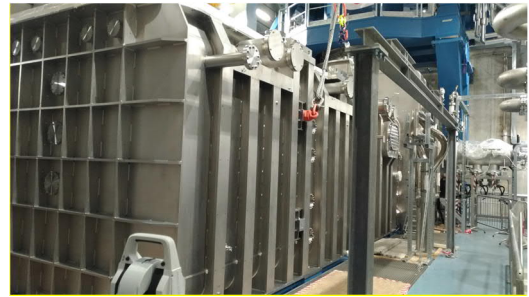
Fig. 6: View of the BLV installed inside MITICA bunker. The leak test of BSV+BLV (part of the SAT) was completed before the coronavirus lockdown.
