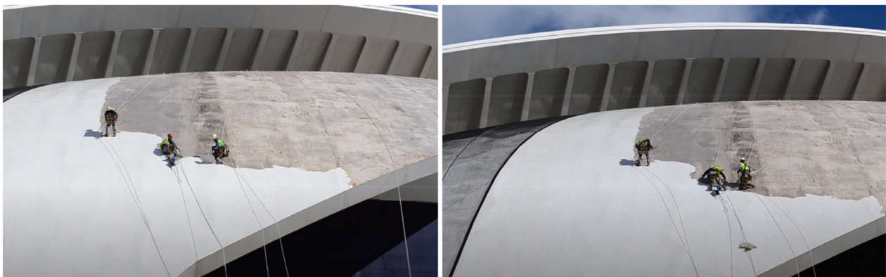
Figure 5. Palau de les Arts Reina Sofia, Valencia (2005). The removal of the trencadís , images from video. Reprinted with permission from Tono Mañes. Copyright 2005 Tono Mañes.
