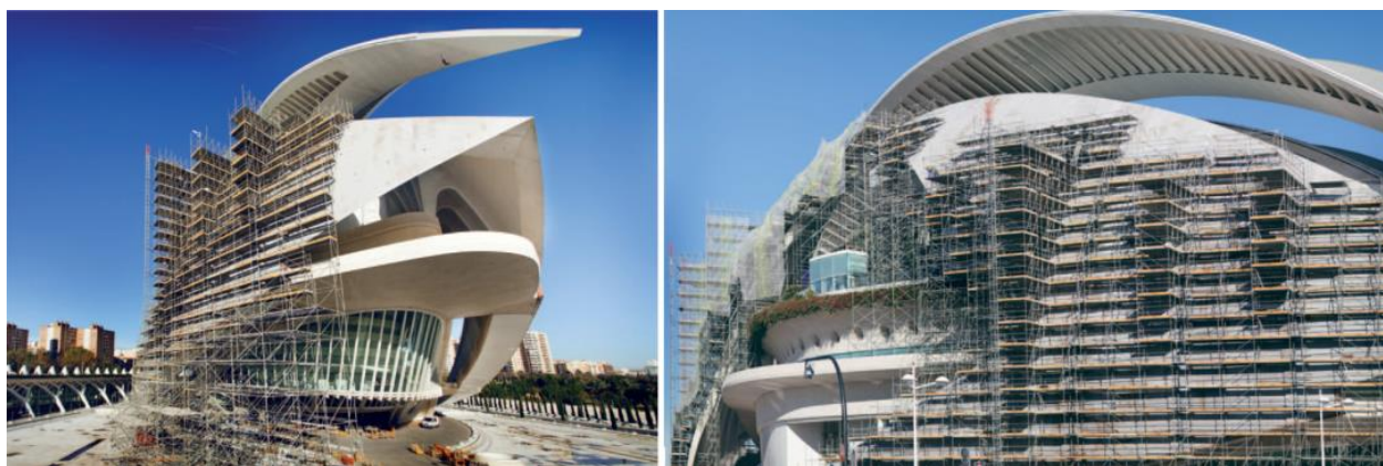
Figure 6. Palau de les Arts Reina Sofia, Valencia (2005). The scaffolding system used for the replacement of the trencadís. Reprinted with permission from ref. [36]. Copyright 2018 Ulma Construction.
