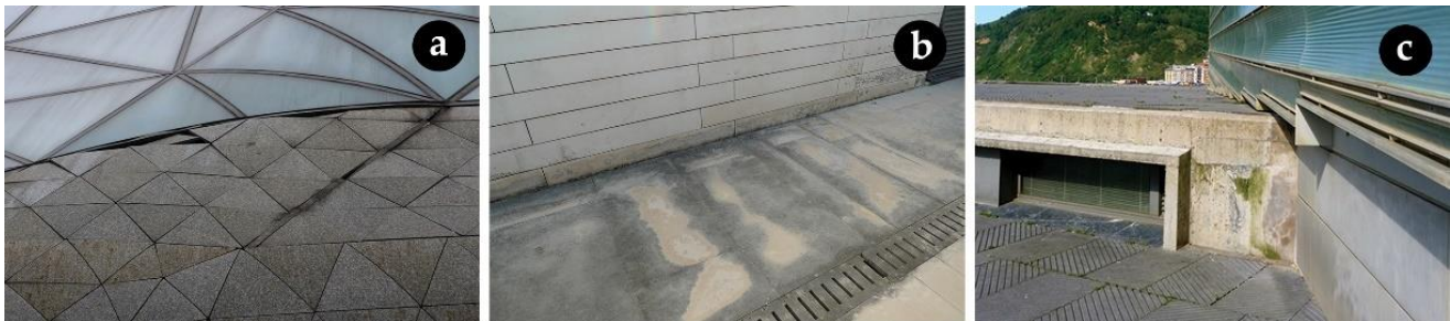
Figure 13. Iconic projects with premature patterns of defects. (a) Guangzhou Opera House (2002–2010) (ph. Cardellicchio, 2017); (b) rectory of the of Nova Universidade in Lisbon (1997–1999) (ph. Tombesi, 2014); (c) concert and convention centre Kursaal in San Sebastian (1996–1999) (ph. Tombesi, 2013).
