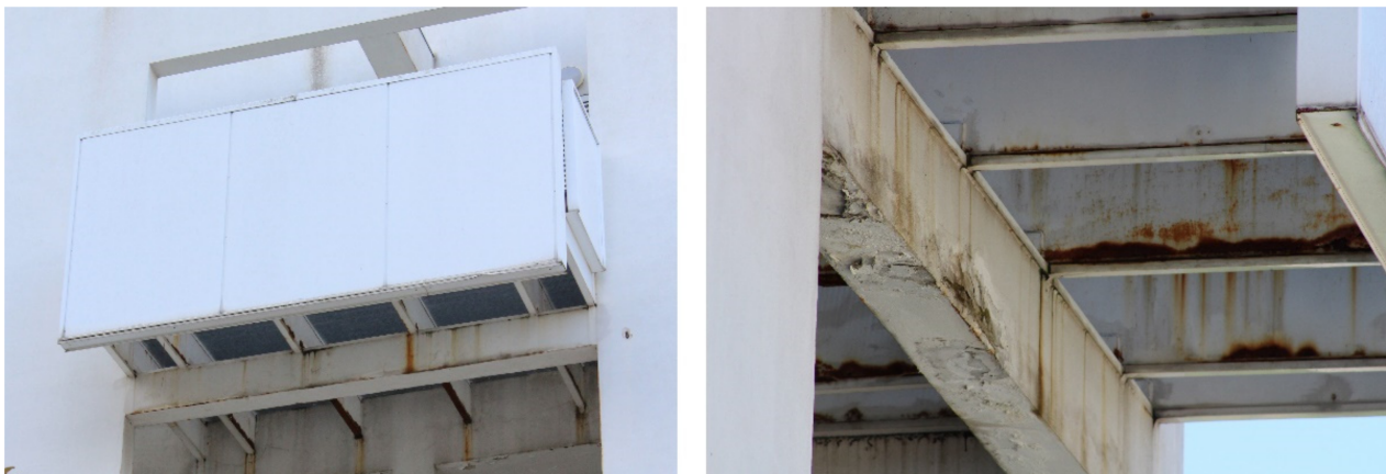
Figure 2. Jubilee Church, Rome (2003). Rusted steel components (ph. Cardellicchio, 2018).
