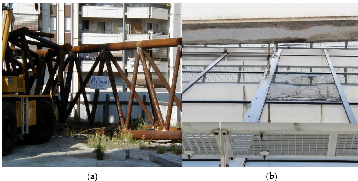
Figure 3. Jubilee Church, Rome (2003): (a) archival picture (26/06/2002) showing part of the steel roof-truss abandoned on site without appropriate cover (ph. Cardellicchio, 2002); (b) broken roof-glass (ph. Cardellicchio, 2018).
