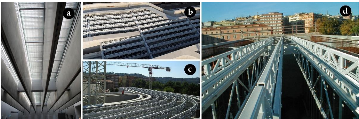
Figure 11. MAXXI, Rome (2010). (a) The roof from the inside (ph. Cardellicchio, 2018). (b–d) Construction pictures of the roof showing the metal blades (courtesy: MAXXI).
