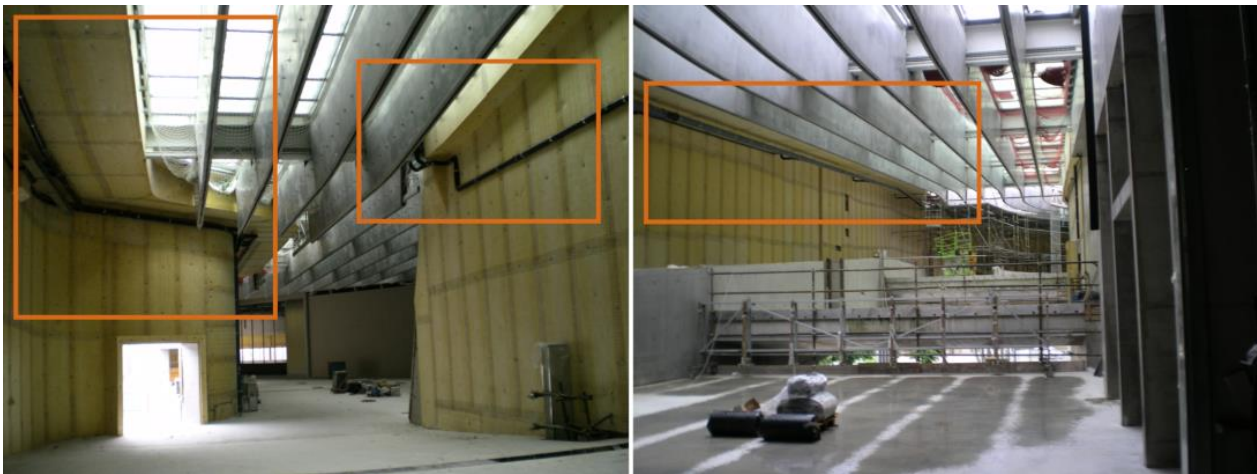
Figure 12. MAXXI, Rome (2010). Construction pictures highlighting the drainage system running inside of the museum (ph. Cardellicchio, 2009).
