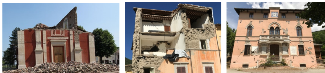
Figure 1. Example of masonry buildings damaged in recent earthquakes in Italy.
