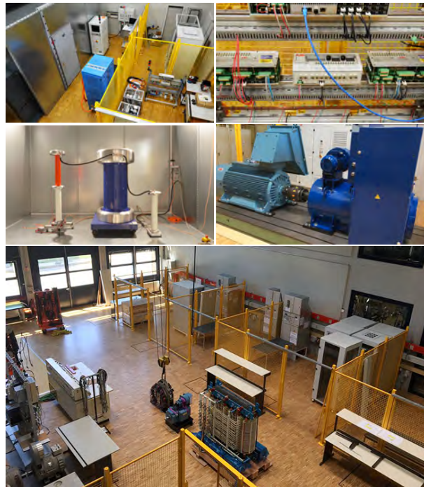
▲ Power Electronics Laboratory
