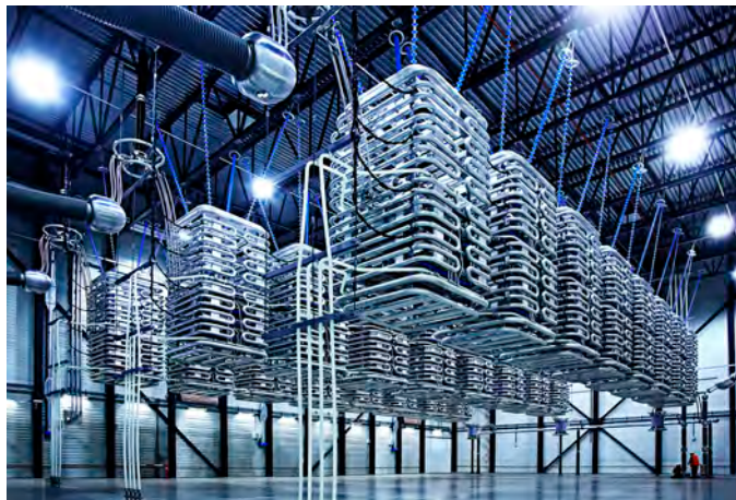
▲ HVDC Light valve hall from ABB.
