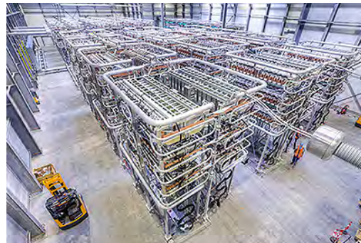
▲ SIEMENS MMC-based HVDC PLUS
