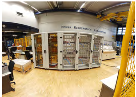
▲ MMC cabinet (hosting ±10kV, 0.5MW converter operating with 96 SMs)
