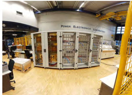
▲ MMC cabinet (hosting \pm 10kV , 0.5MW converter operating with 96 SMs)
