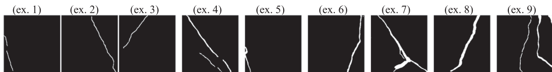
Fig. 13. Segmented cracks on examples images in Fig. 10(a) by TernaNet (model B).
