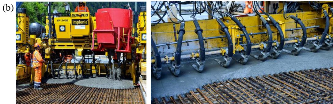
Figure 2 Rehabilitation using UHPFRC: (a) Chillon viaduct after strengthening; (b) UHPFRC casting finisher
