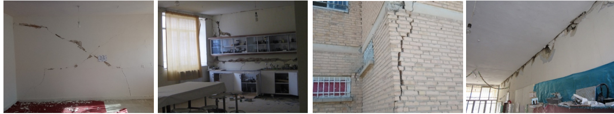
(a) Diagonal crack of walls (b) Concentrated cracks (c) Separation of walls (d) Sliding of the roof
