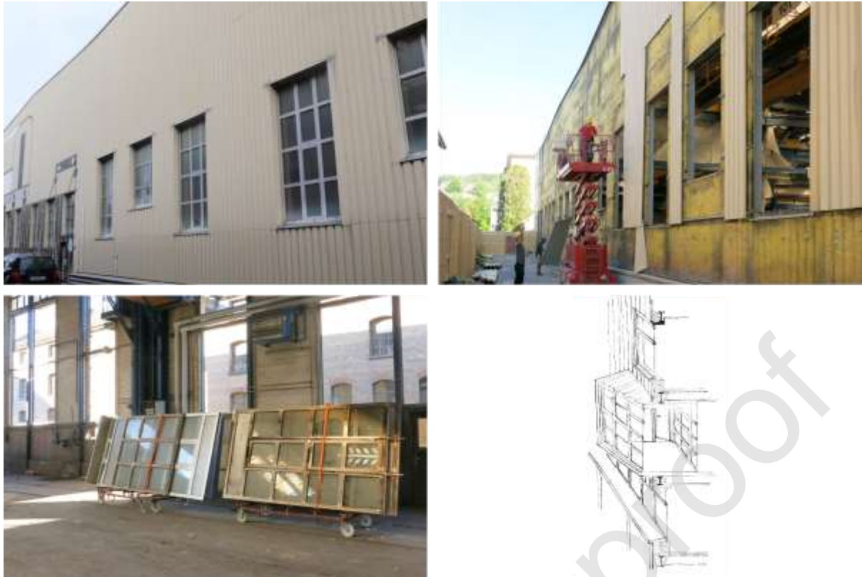
Figure 7: (a) Window frames reused from the demolition site, (b) dismantling of window frames, (c) storage, (d) adapted design for use of these window frames in K.118 (Baubiuro in situ, 2018)
