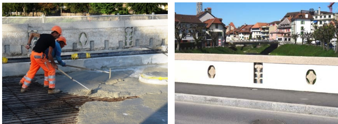
Figure 13. Casting of the UHPFRC on the deck slab; the UHPFRC layer incorporates steel rebars. Restored decorative elements of the parapets.
