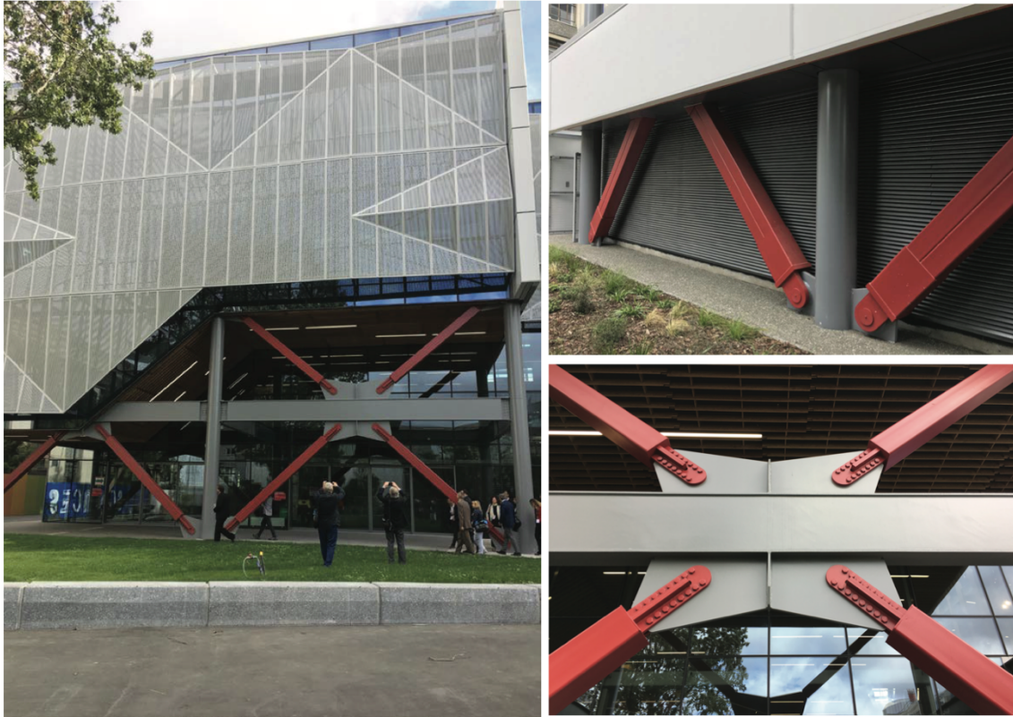
Figure 16. Buckling-restrained braced frames including typical bracing connections (photos from University of Canterbury campus, New Zealand, courtesy of Prof. Dr. D. Lignos)
