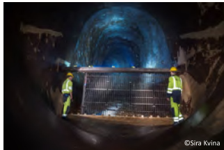
Trash rack in the Duge power plant
