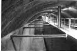
Settling Basin of KWGO
