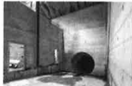
Forebay tank of KWGO
