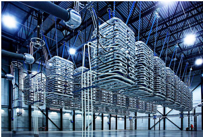
▶ HVDC Light valve hall from ABB.
