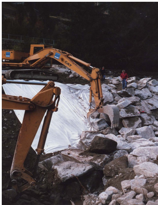
Fig. 1. Riprap with blocks of 4–4.5 t being individually placed by a machine on a geotextile serving as a filter. (Image by A. J. Schleiss.)
