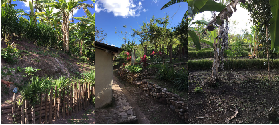
Fig. 5 Soil-bioengineering measures for slope stabilization in Honduras. From left to right: wattle fence, dry wall of crude stones, and berm construction stabilized with vetiver. (Silvia Hostettler, EPFL)
