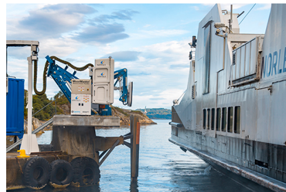
▲ WARTSILA wireless coastal ferry MW charger (Source: www.wartsila.com )
