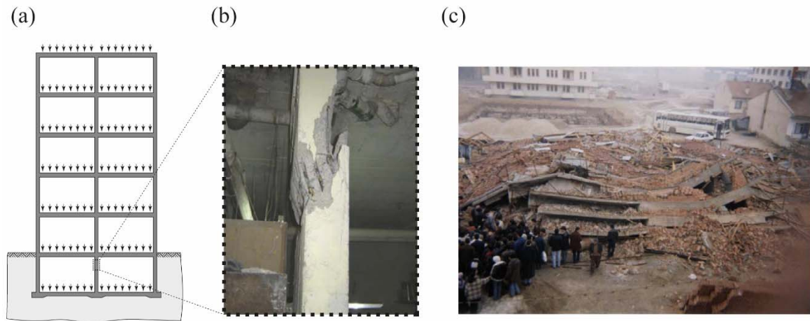
Fig. 2-3 Zumrut apartment building in Turkey: (a) Structural system, (b) heavy damage in the basement columns due to nonlinear creep, and (c) Collapse aftermath (taken from (Kaltakci et al. 2007))
