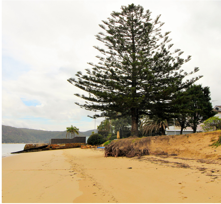
Figure 33: The northern part of Sandy Beach : an impressive dune scarp in the foreground and in the background, the seawall built around Sand Point.
